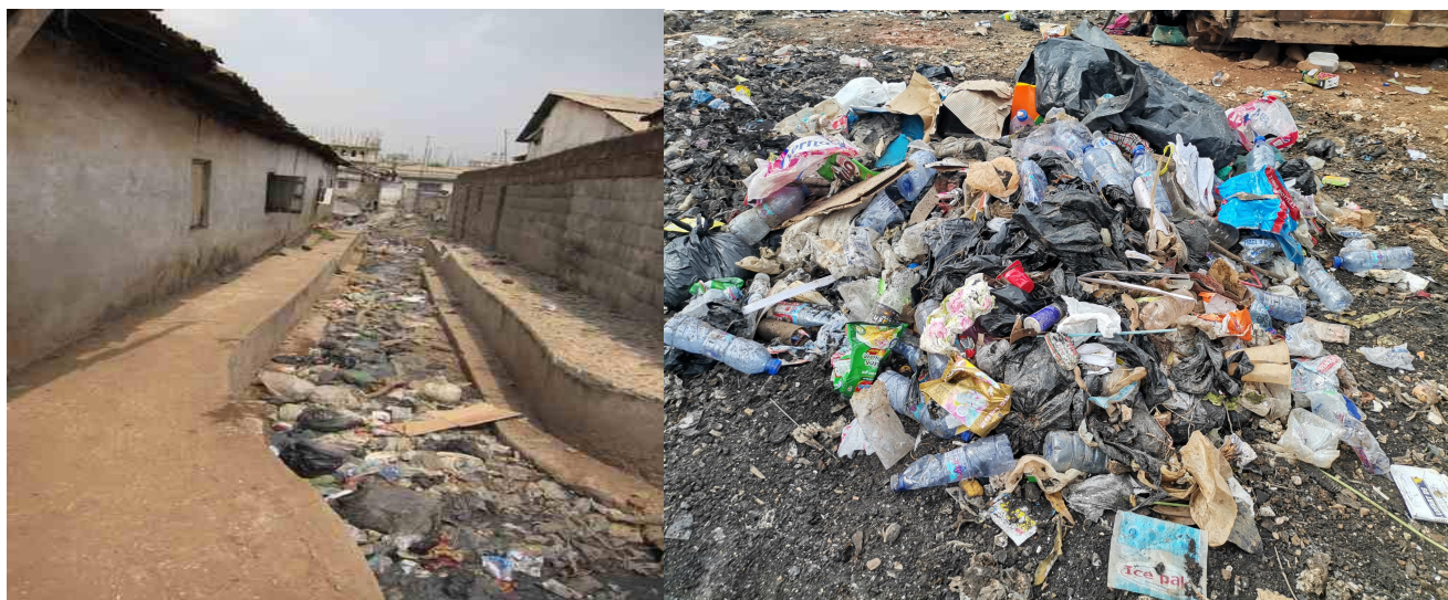
Figure 1: Choked gutter with plastic bottles and landfill site at Effiakuma New Site -Takoradi
